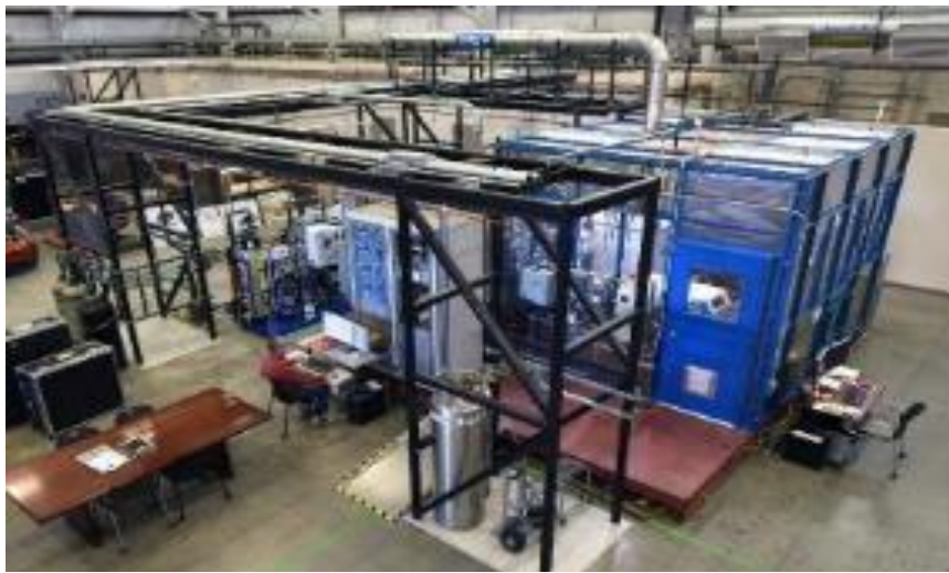
High Temperature Electrolysis Facility (INL)
